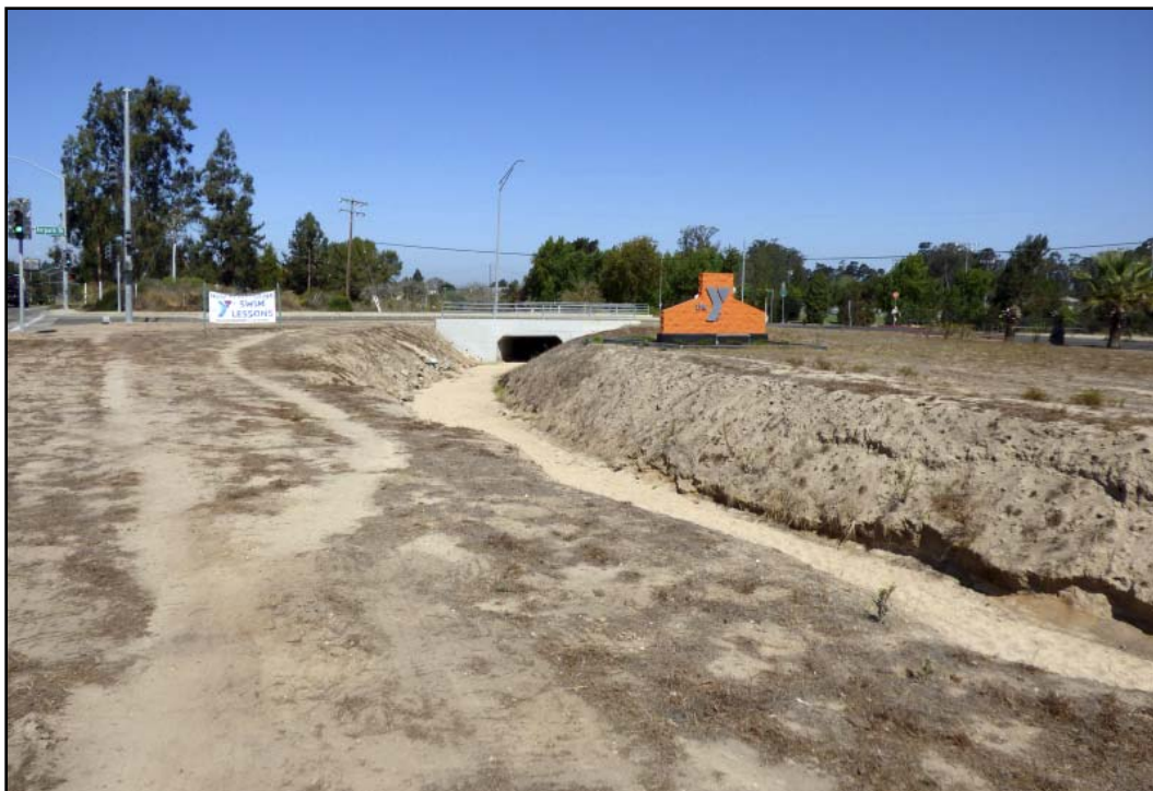
PHOTOGRAPH 8 Views of Hagerman Drive Bridge Over SMAD Looking Northwest Near YMCA Entrance and Monument Sign
