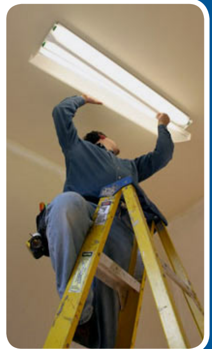
The lighting replacements alone are saving approximately 2.1 million kwh/year Countywide.
