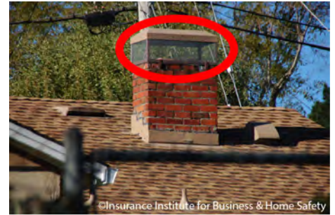
A spark arrestor at the top of a chimney.
