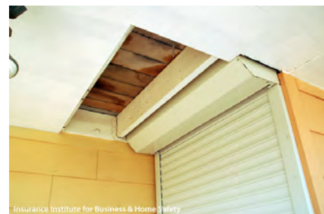
A horizontal enclosure, such as that shown here, can result in moisture-related degradation of wood and metal fasteners when deck boards are used.
