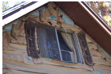
Deformed vinyl siding from a radiant heat exposure from a nearby burning home. Source: Stephen L. Quarles
