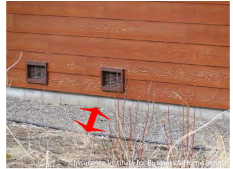
A noncombustible zone around a home in the Lake Tahoe Basin. In this case, requirements related to water runoff and protection from wildfire align.
