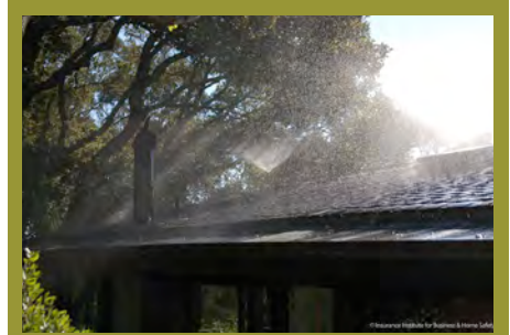
Photo 1. Roof mounted sprinkler.
