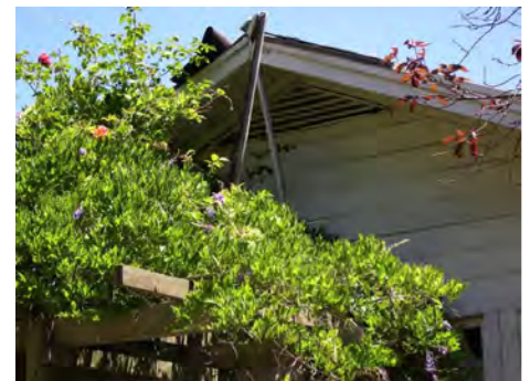
Vegetation growing over a trellis structure. If ignited, flames would impinge on the side of the house, including the nearby gable end vent. Source: Stephen L. Quarles
