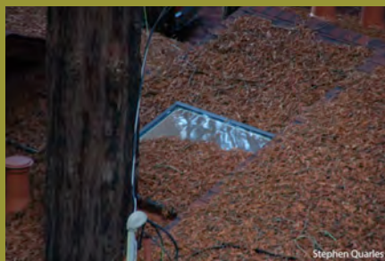
Photo 1. Accumulation of vegetative debris on top of a glass-type skylight on a low-slope roof.
