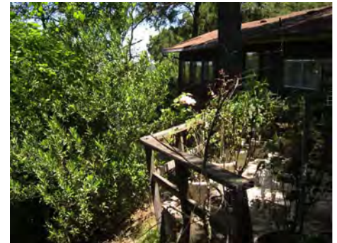
The defensible space on this property could be improved by removing vegetation to minimize the opportunity for fire to burn directly to the home. Source: Stephen L. Quarles
