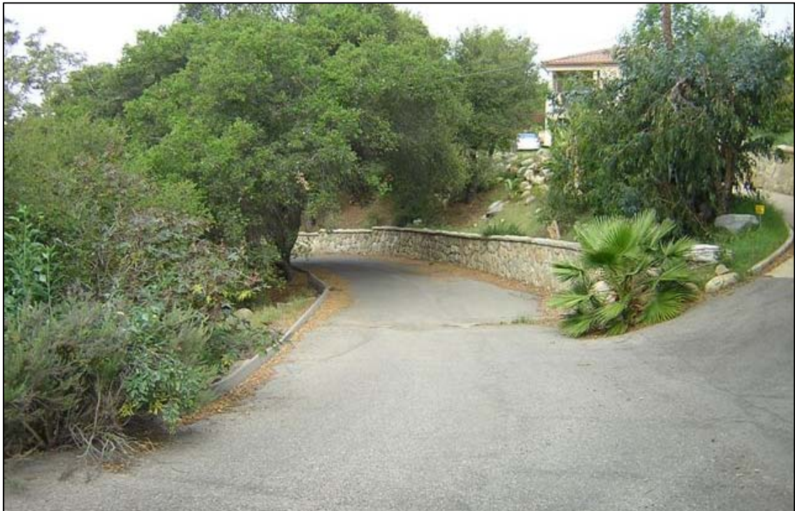
Lower portion of San Antonio Creek Road adjacent to eastern driveway of Fee Residence. The road is a minimum of 20 feet wide in this section. Roadside vegetation could be trimmed to maintain adequate clearance for emergency access.
