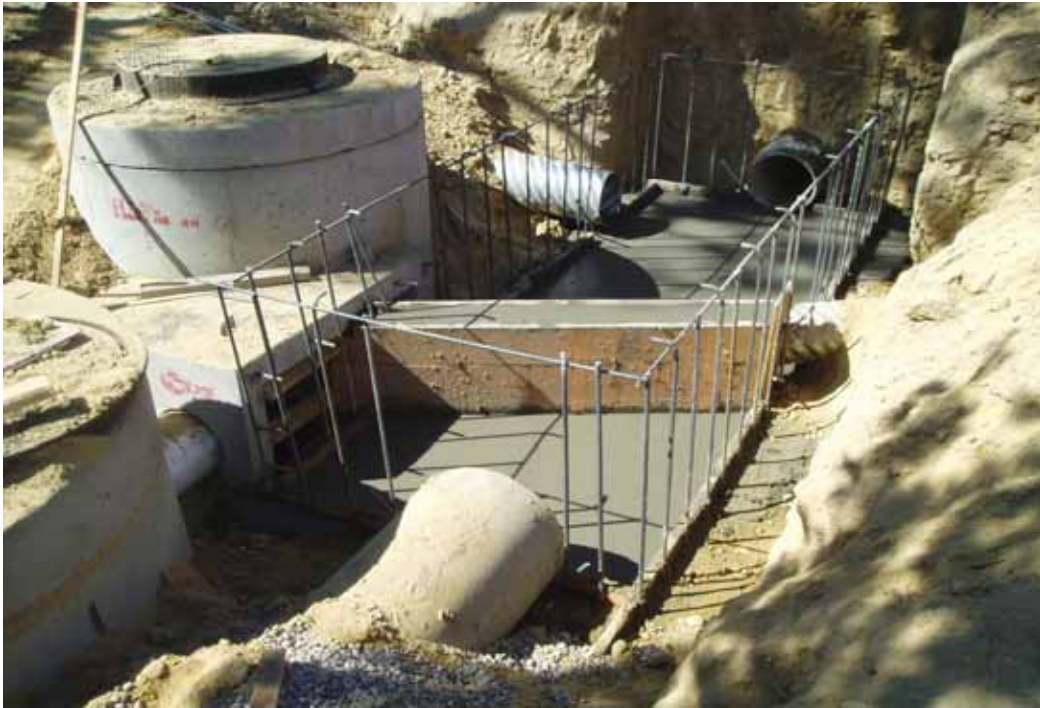
Diversion structure under construction with portion of CDS Clarifier unit visible at left back and portion of low flow water sump visible in left foreground.
