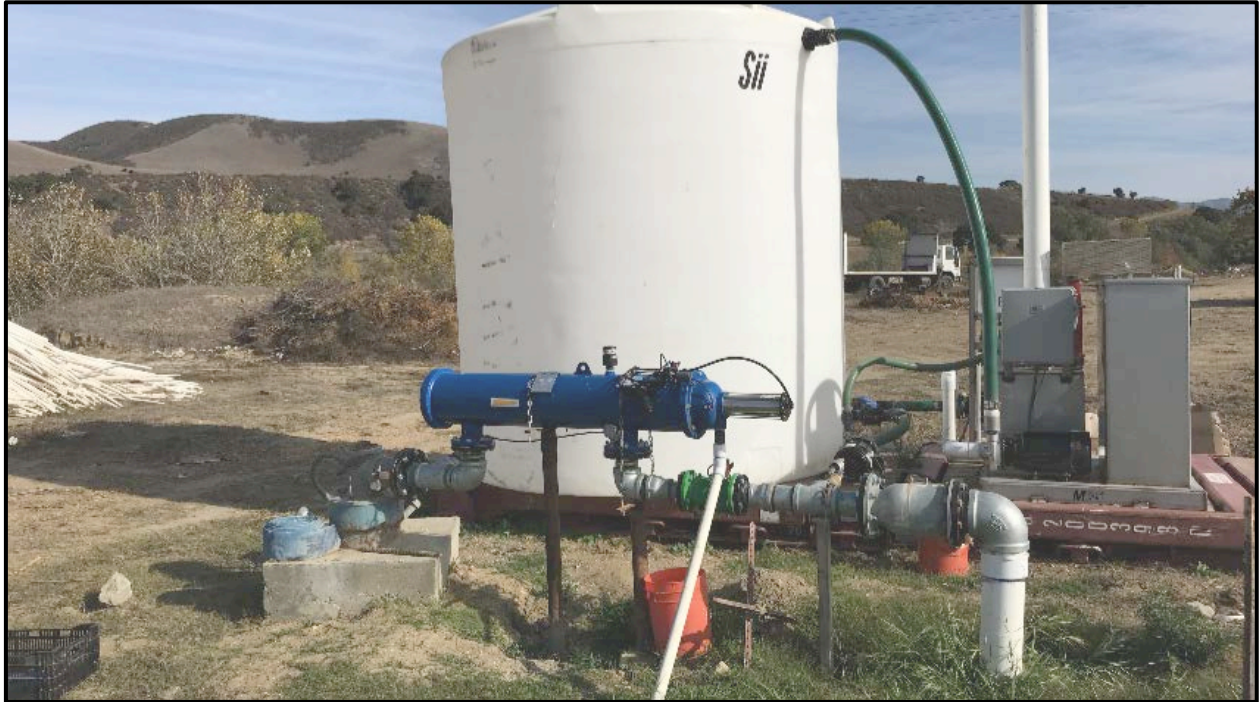
Photo 1. The shallow alluvial water well at 5645 Santa Rosa Road.
