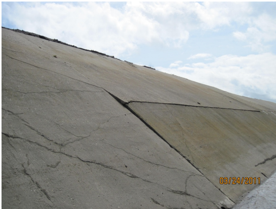
A portion of the concrete lined Rodeo/ San Pasqual Channel in need of repair
