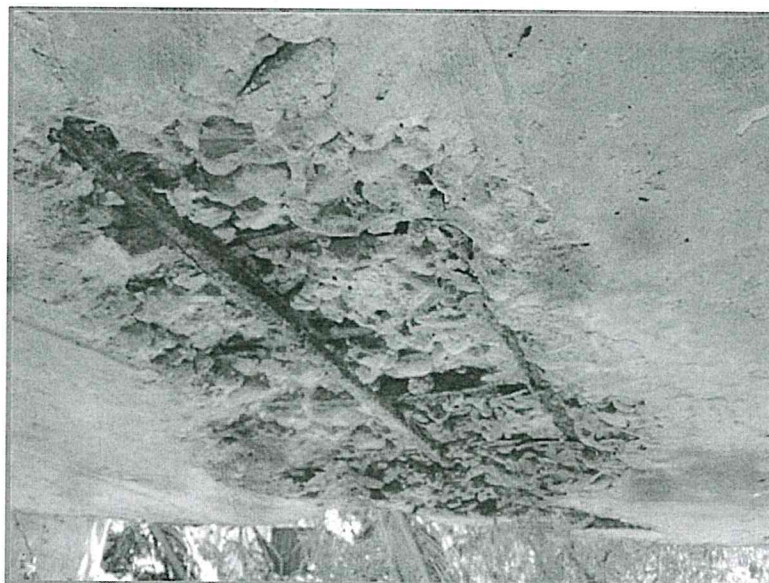
Photo 3: Spalling on roof of culvert
