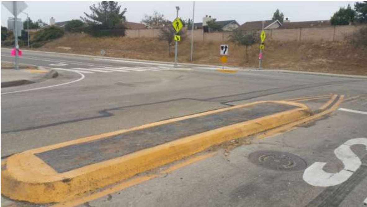
Typical intersection of road surface to be treated on Union Valley Parkway
