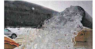
Water, Recycled Water, and Sewer Pipelines
