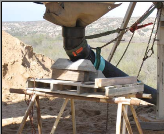
2 nd unders discharge to Eagle dehydrator
