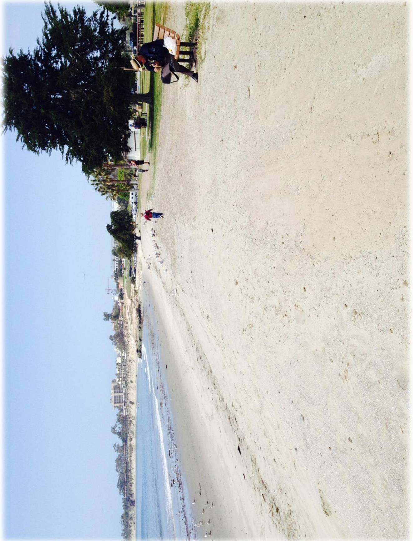
Repair area facing east from east end point of existing permitted revetment (under CDP 4-14-0687)
