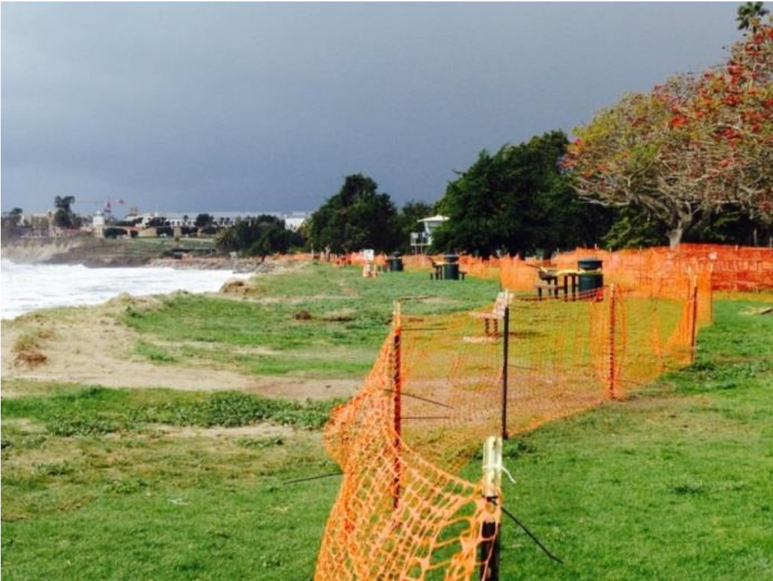
Sinkholes and erosion aspect west (Mar 7)
