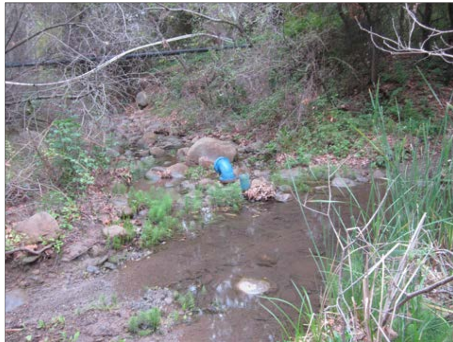
Photo 5: View of unpaved low water crossing looking south at pipe blow off
