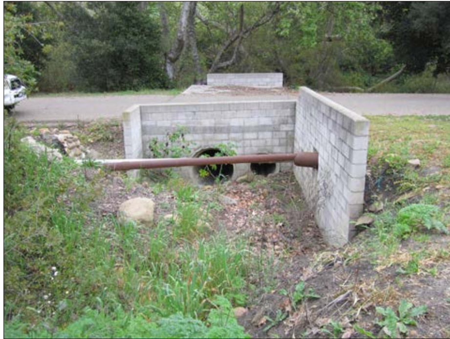
Photo 1: View of agriculture drain structure/culvert on west side of access road (potential bioretention basin location)
