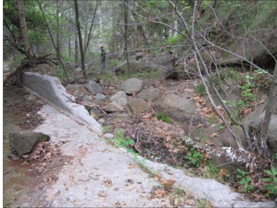
Photo 2: View of upstream end of creek diversion channel at broken wall and start of proposed secondary channel
