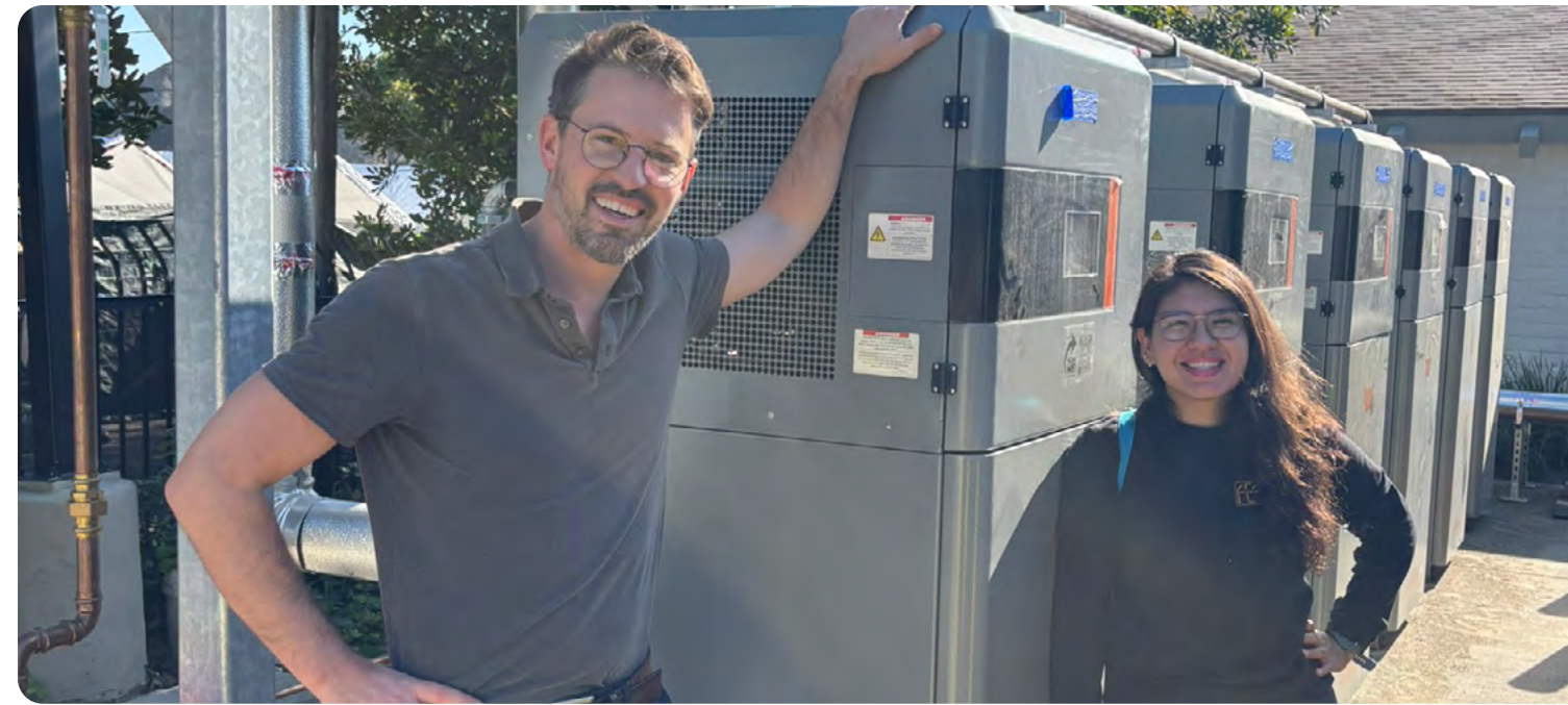
America Diaz (3C-REN Technical Assistant) and David Ross (Senior Project Manager from Ventura Housing, the housing authority of the City of Ventura) in front of Valentine Road Apartment's central heat pump water heating system.
