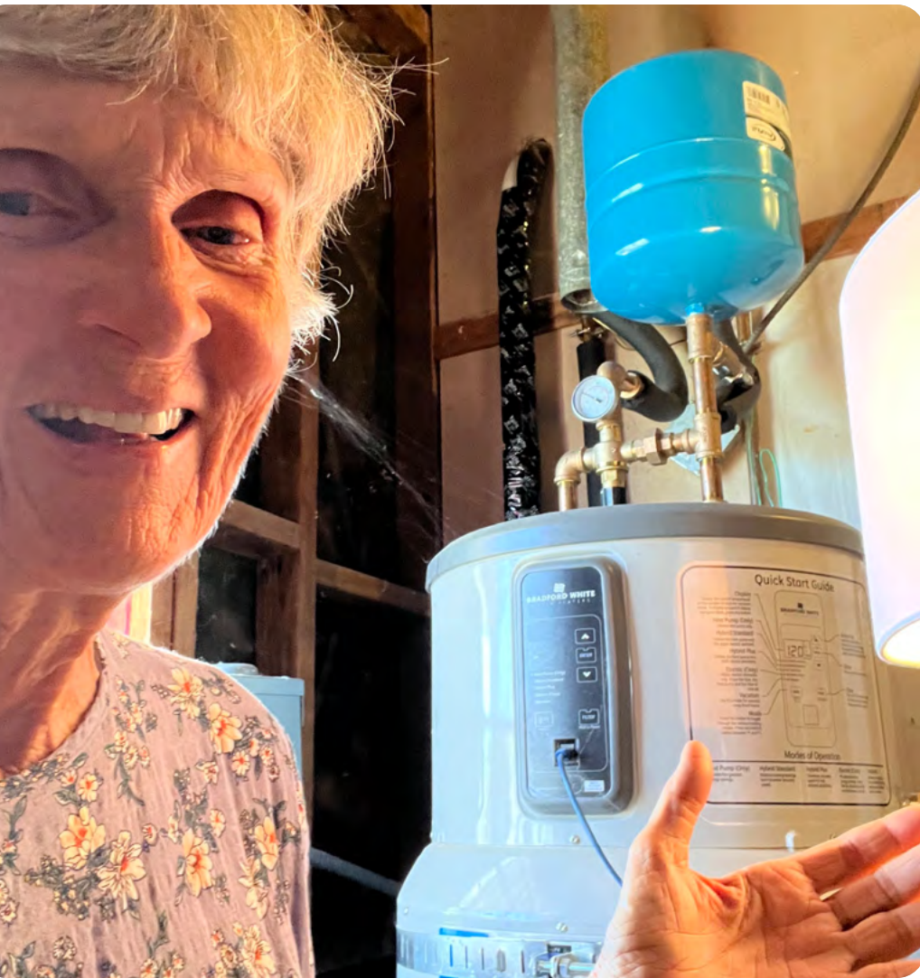
Karen Mortensen stands in her garage and shows off her heat pump water heater.
