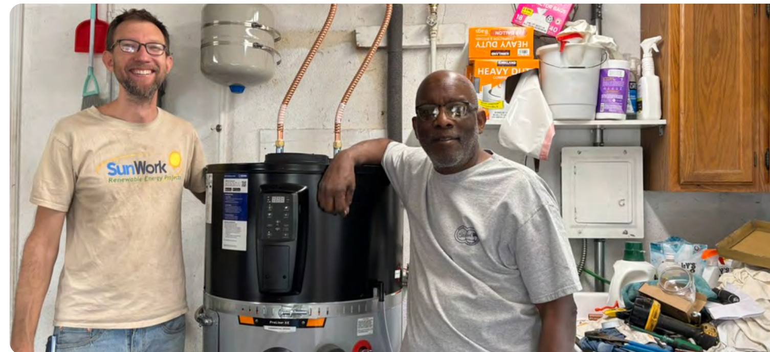
Reuben Veek of SunWork trains workforce program participant Vernon Staples how to install a heat pump water heater at a home in Ojai.
