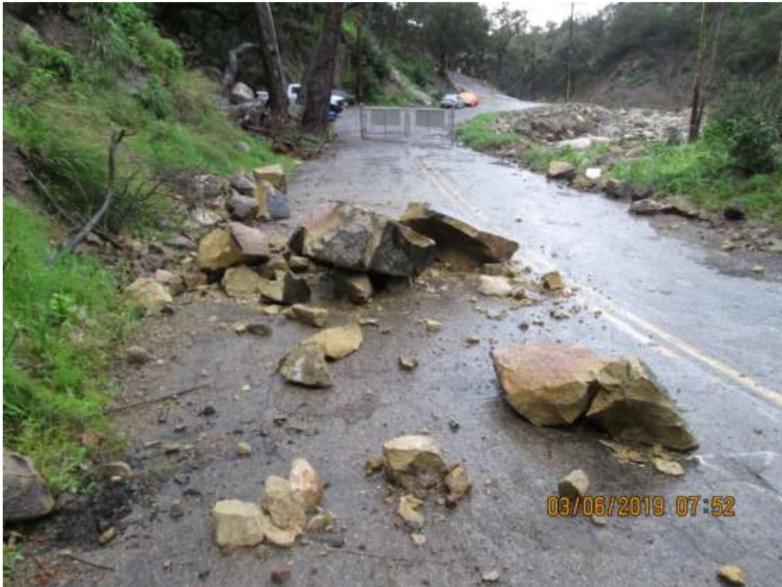
View of East Mountain Drive, looking south. The embankment slope above the roadway was denuded of vegetation as a result of the Thomas Fire and experienced rockfall events as a result of the fire and subsequent intense rainfall events. Recent Rockfall from 2019 shown.
