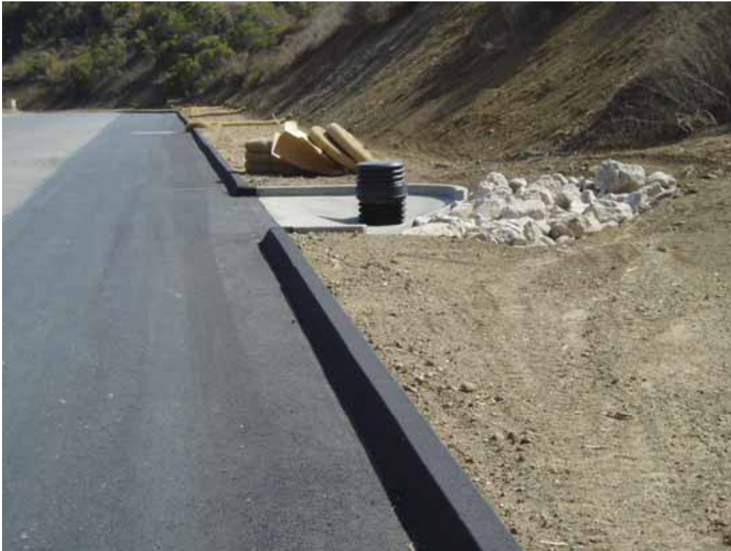
View of completed project with drainage inlet at center right and road reinstatement and widening over the new 48-inch diameter storm drain.
