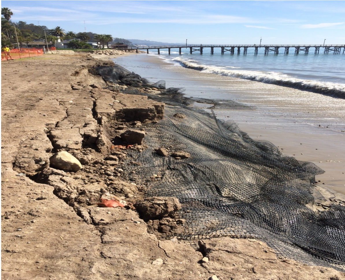
February 2017 Geotextile Damage
