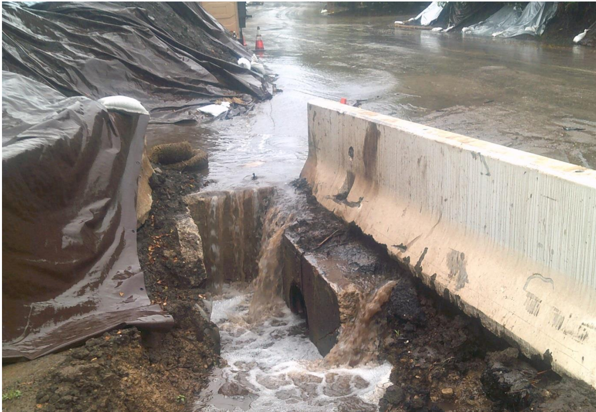
View of Santa Isabel Lane, looking north from N Jameson Lane. The storm drain inlet shown was heavily damaged during the debris flow event, which destroyed the inlet cover and the surrounding asphalt concrete dike, as well as filled the culvert pipes with debris. Project proposes to reconstruct the damaged drainage inlet structure, as well as damaged culvert pipes connecting to the flood control drainage system. Photo is from March 2018.
