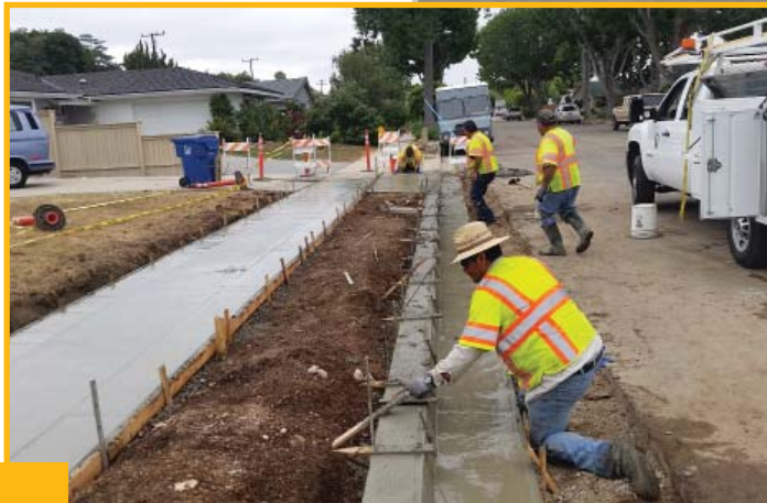
Photo to the right: Recent concrete work performed by our crews on San Lucas Way.
