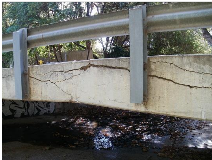
Existing Fernald Point Lane Br. No. 51C-0137 over Romero Creek, looking easterly
