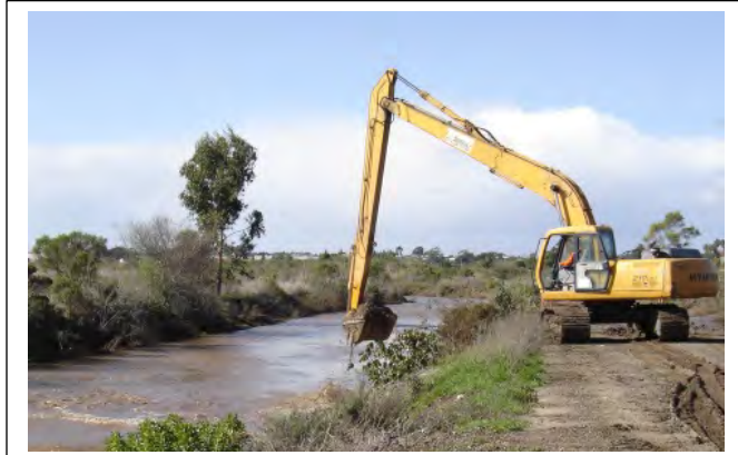
The Flood Control District maintains over 200 miles of major channels to ensure conveyance of peak flows to prevent damaging flooding in communities throughout the county.
