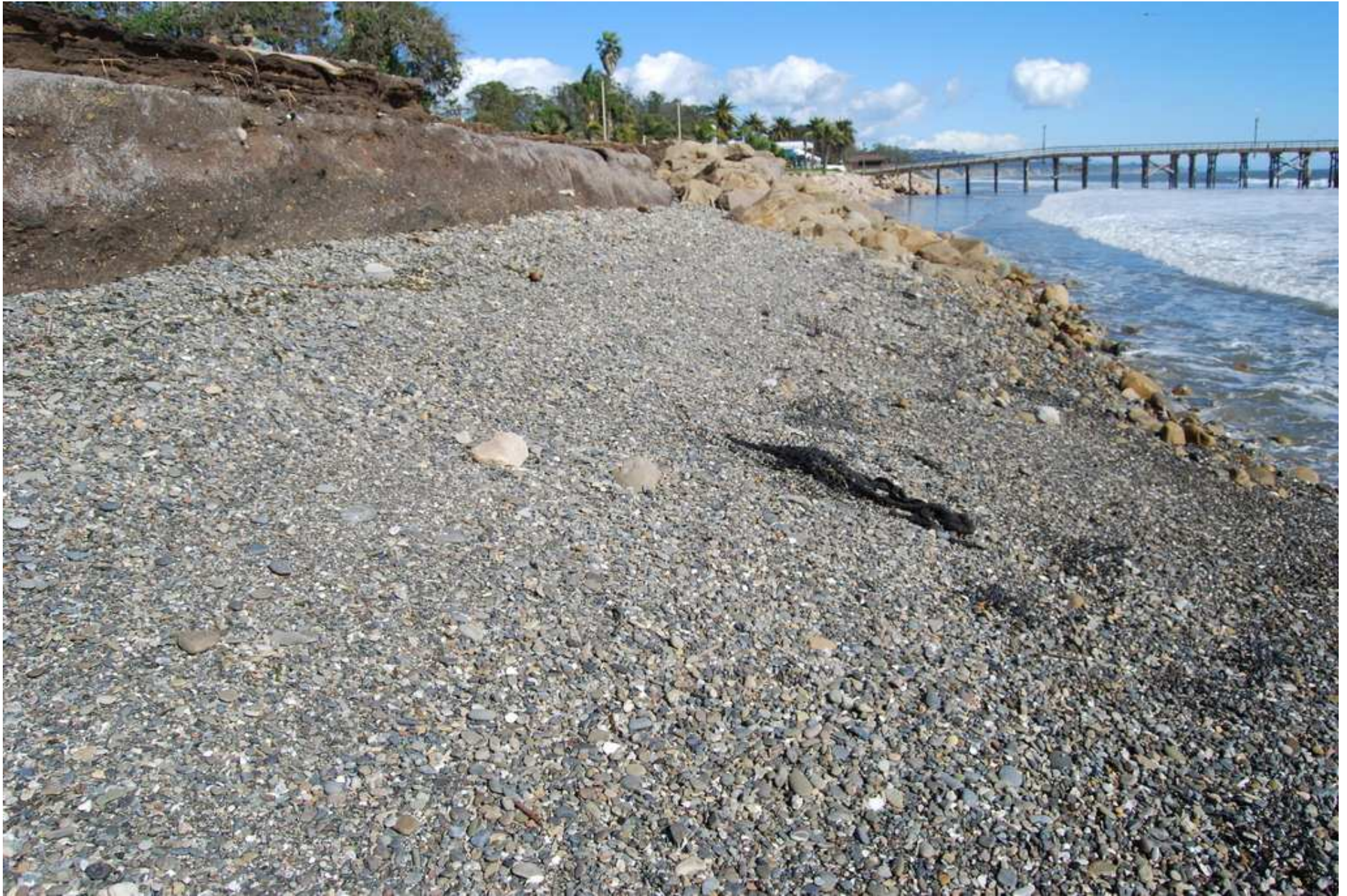
Several hundred tons of wave-driven cobble fills the gap left by the shredded geotextile structure.
