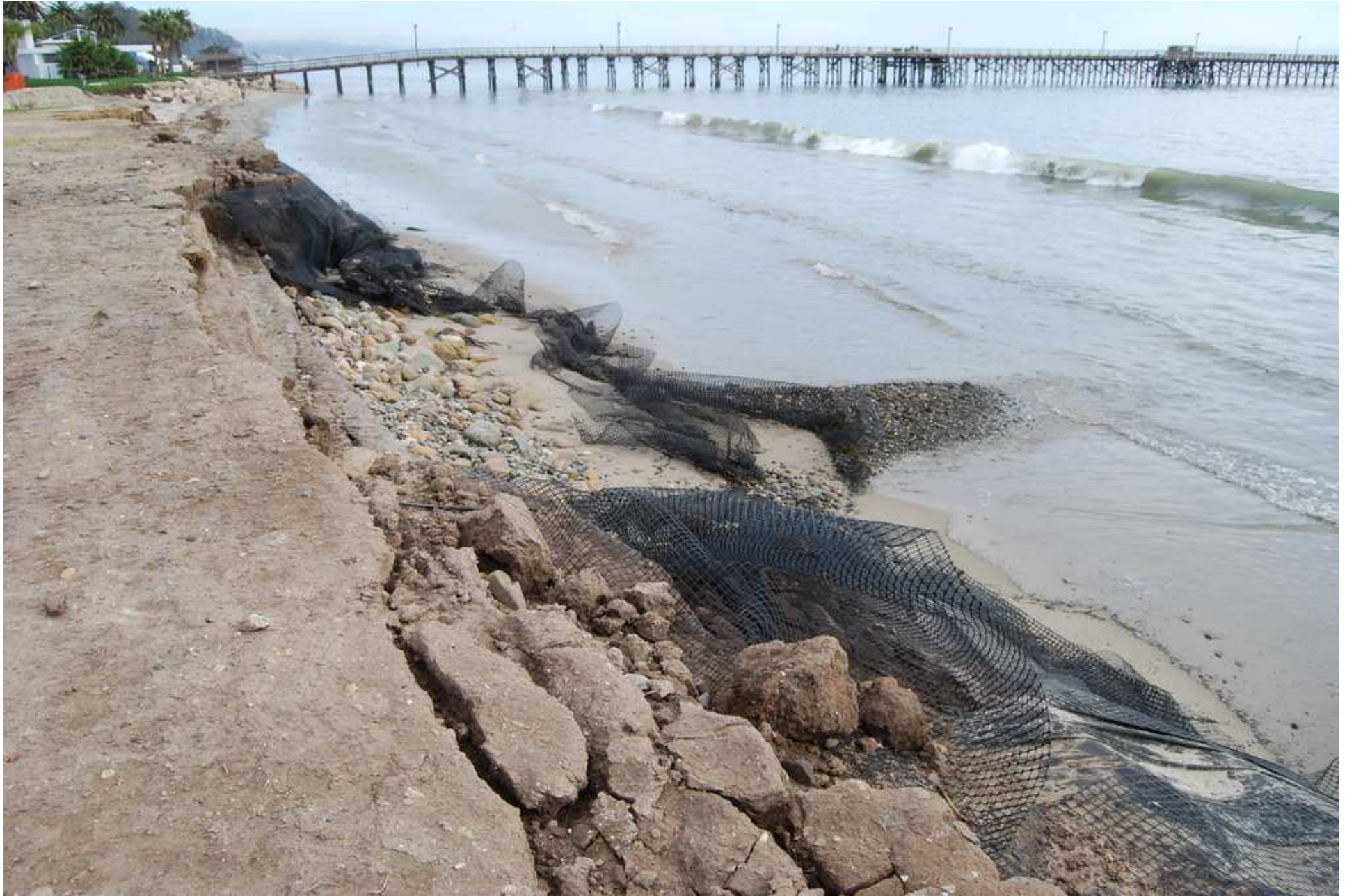
Expensive, ill-advised geotextile structure, shredded by waves, deposits a trivial amount of cobble on the beach. February 15, 2017.
