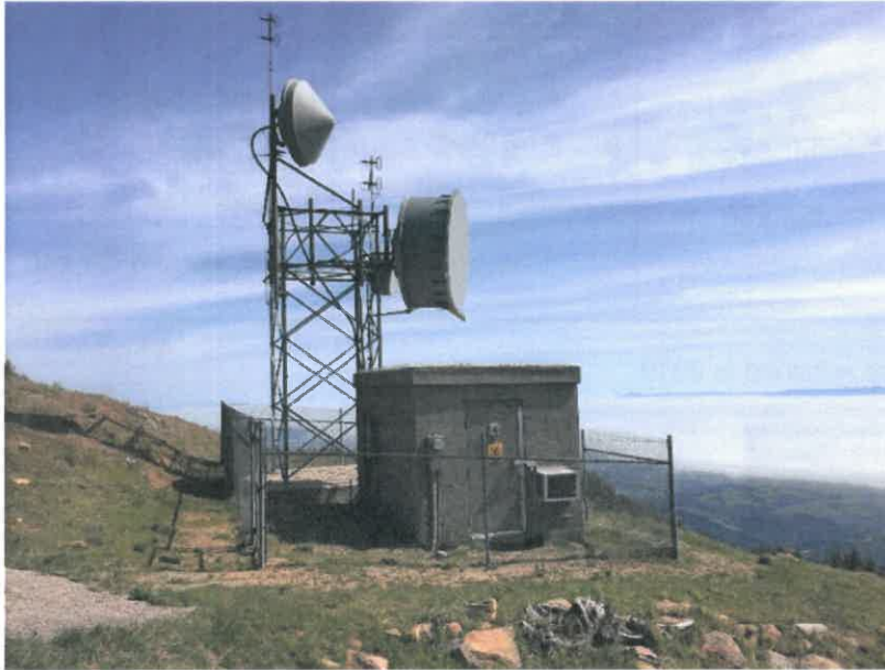
Facility #1 Exxon Mobil
