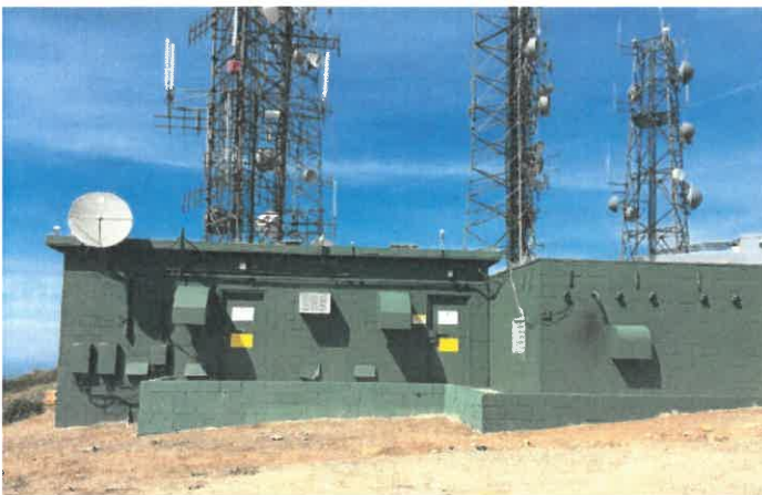
Facility #11 American Tower, LP building & tower (left)
