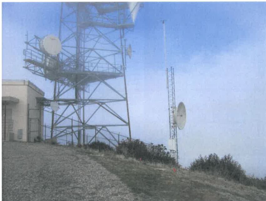
Facility #6 Regents of the Univ. of CA tower (right) and Facility #7 Frontier California Inc (left)
