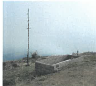
FS fuel surround & SBC pole #3
