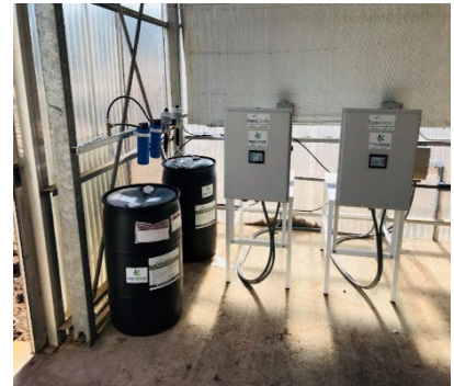
Odor Pumping Equipment
