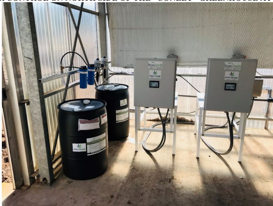
Odor control pumping systems in a greenhouse
