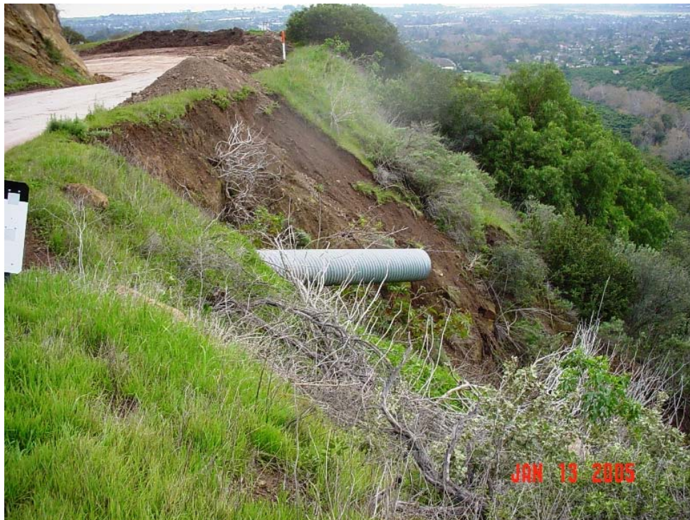
San Marcos Storm Damage Repair Site at Mile Post 1.7 north from Cathedral Oaks Rd.
