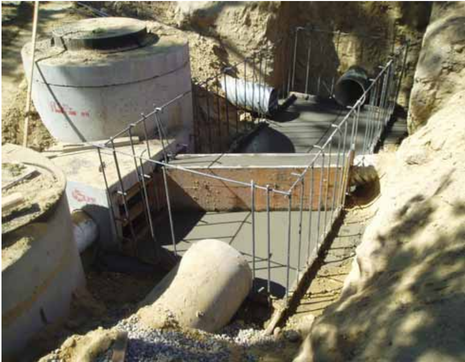
Diversion structure under construction with portion of CDS Clarifier unit visible at left back and portion of low flow water sump visible in left foreground.
