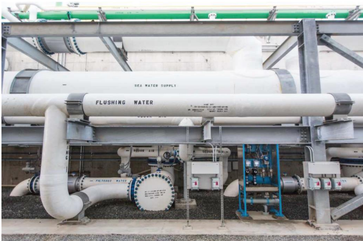
Pictured: Media filter system
