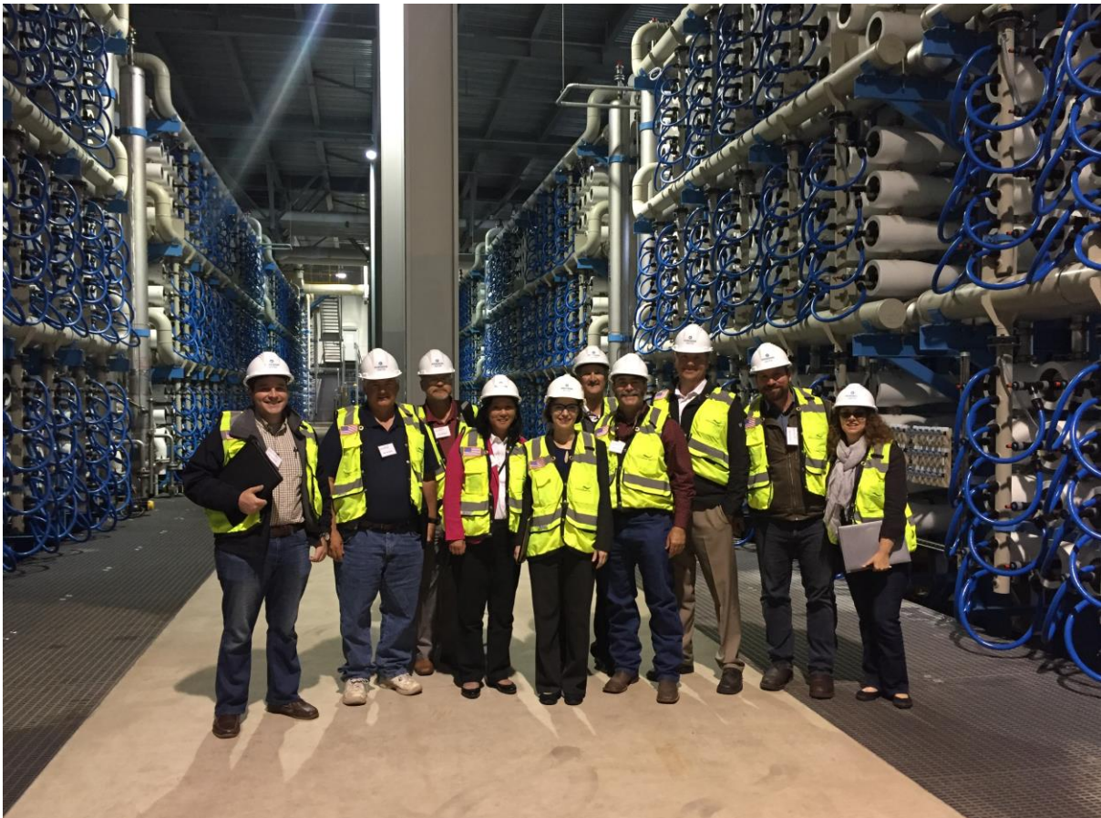
Pictured: Staff with reverse osmosis array
