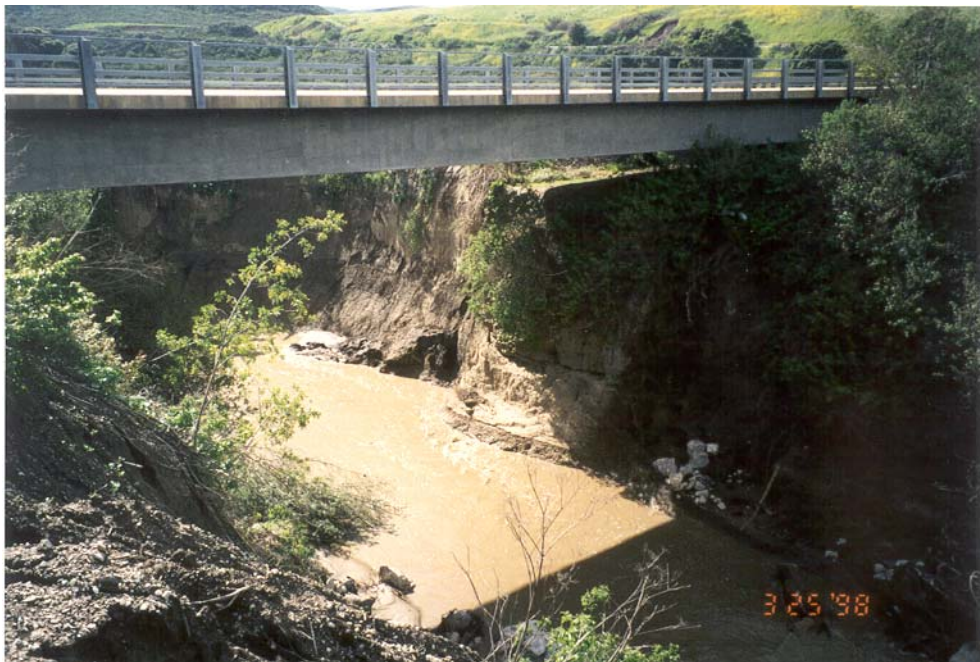
Photo: Existing Salsipuedes Creek embankment conditions at Santa Rosa Road Bridge 51C-020
