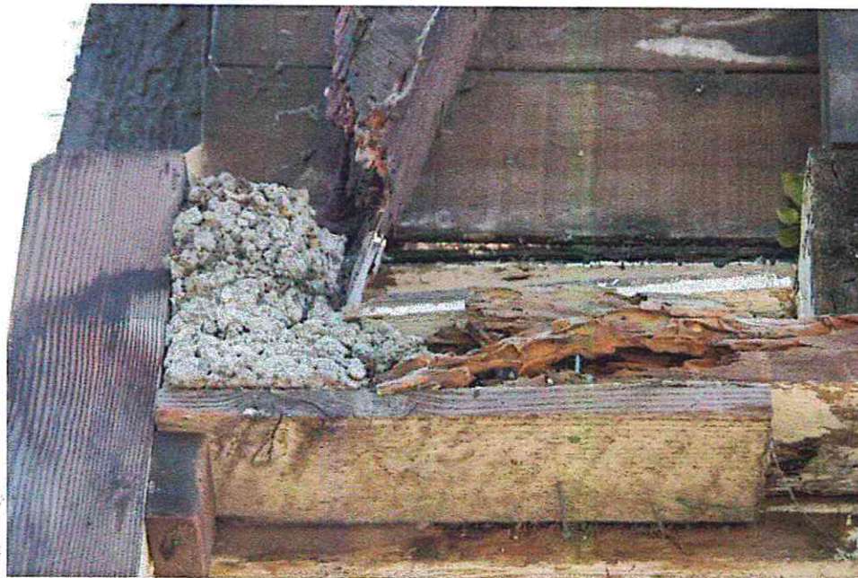
Photo 7 : Rot at key structural connection
