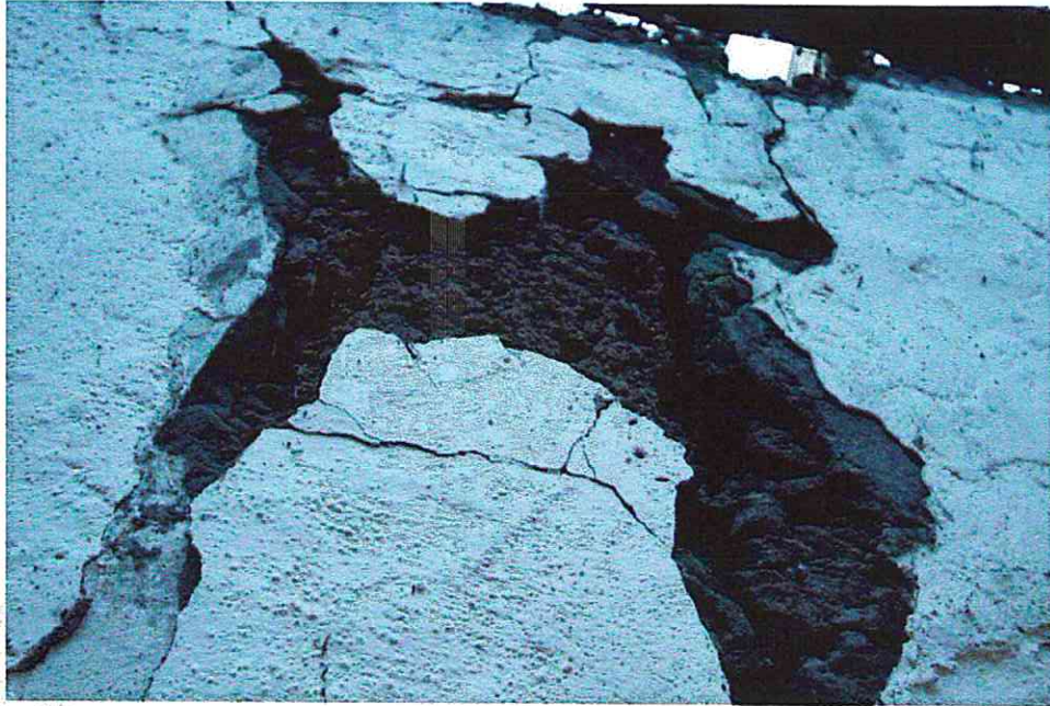
Photo 3 : Deep Erosion at top perimeter of wall line due to water intrusion
