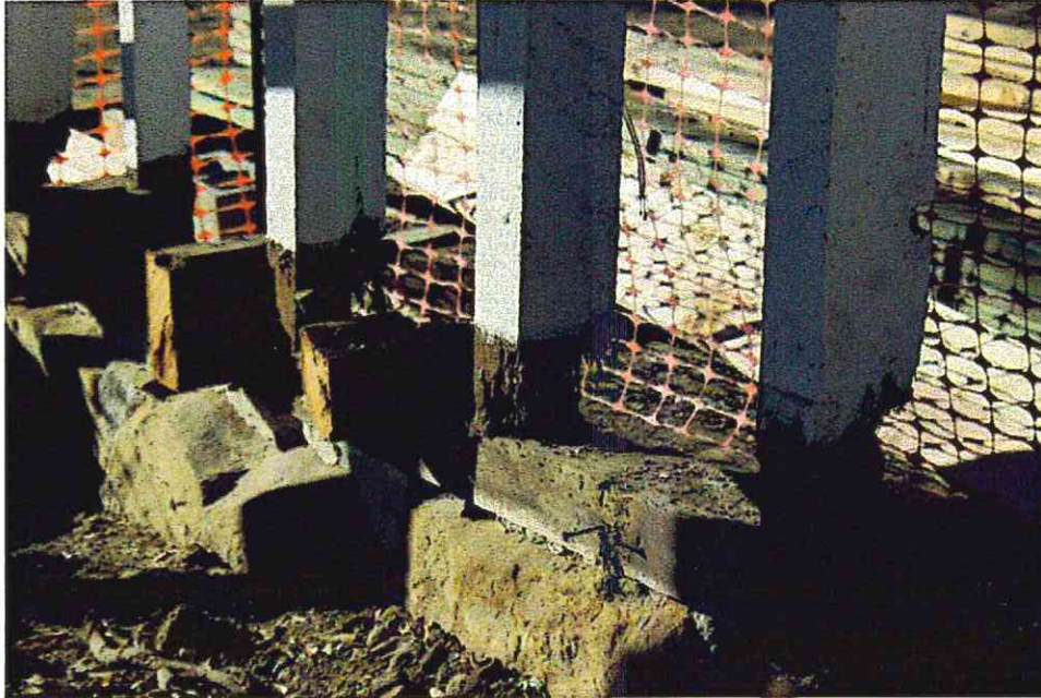
Photo 5 : Vertical support posts completely rotted at sill plate
