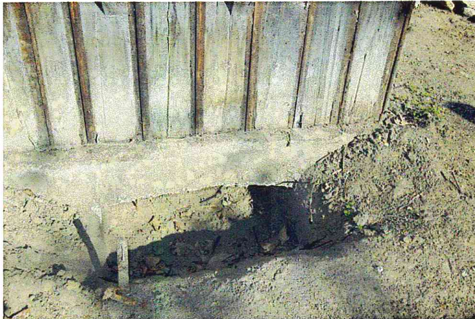
Photo 10: Excavation at perimeter of slab at Cottage showing the absence of a footing
