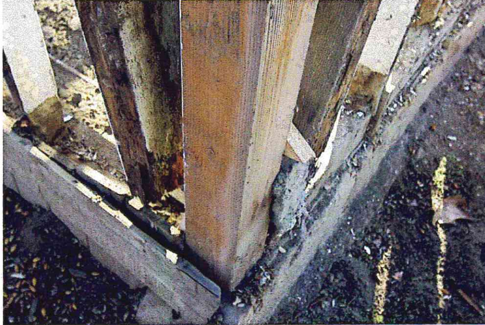
Photo 9: Stone Foundation at Tower on right, earth to wood contact on left
