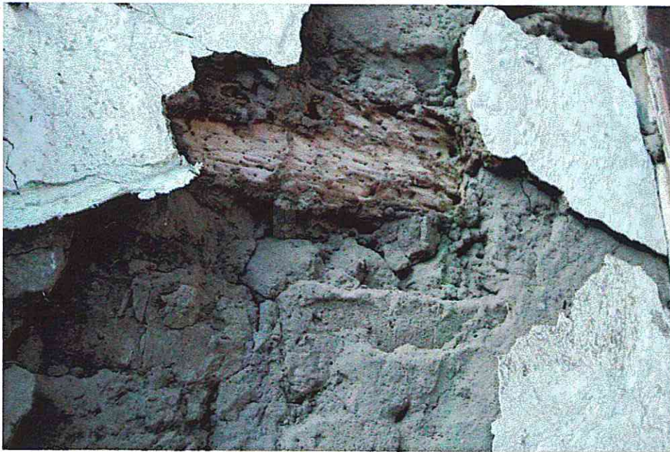
Photo 4 : Pest Intrusion typical at all wood to adobe interface
