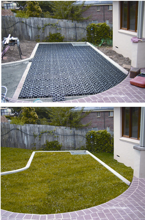
Figure 3.9 – Grasscell Used to Manage Stormwater Runoff
