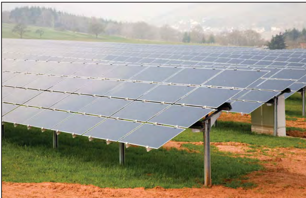
Example Photovoltaic Pole-Mount Arrays, View 1.
