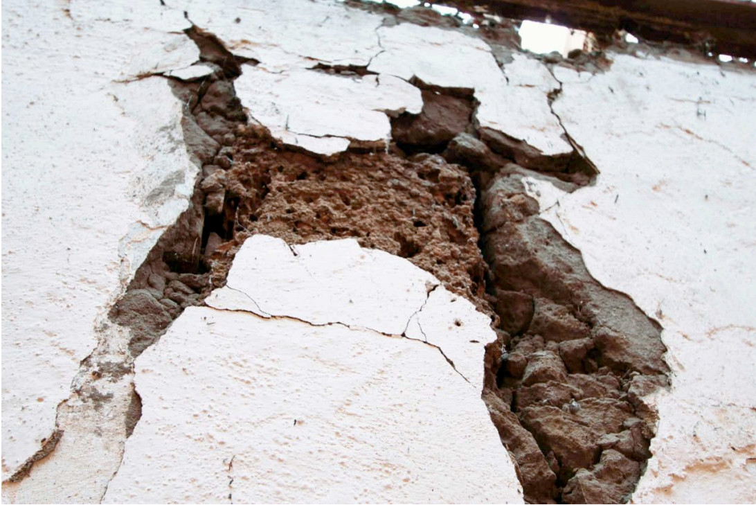
Plate 11. Upper adobe wall showing crumbling blocks. November 2013.
