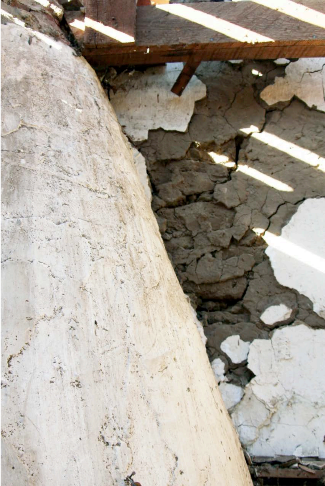
Plate 13. Crumbling blocks adjacent to fireplace. November 2013.
