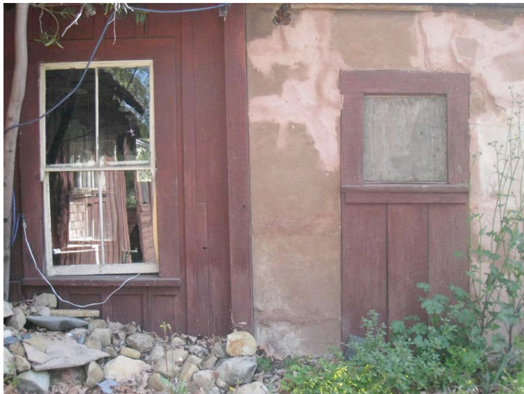
Plate 2. Detail of window at left to be removed and re-used and the opening enlarged for the new front entry. Facing east. April 2010. A. C. Cole
