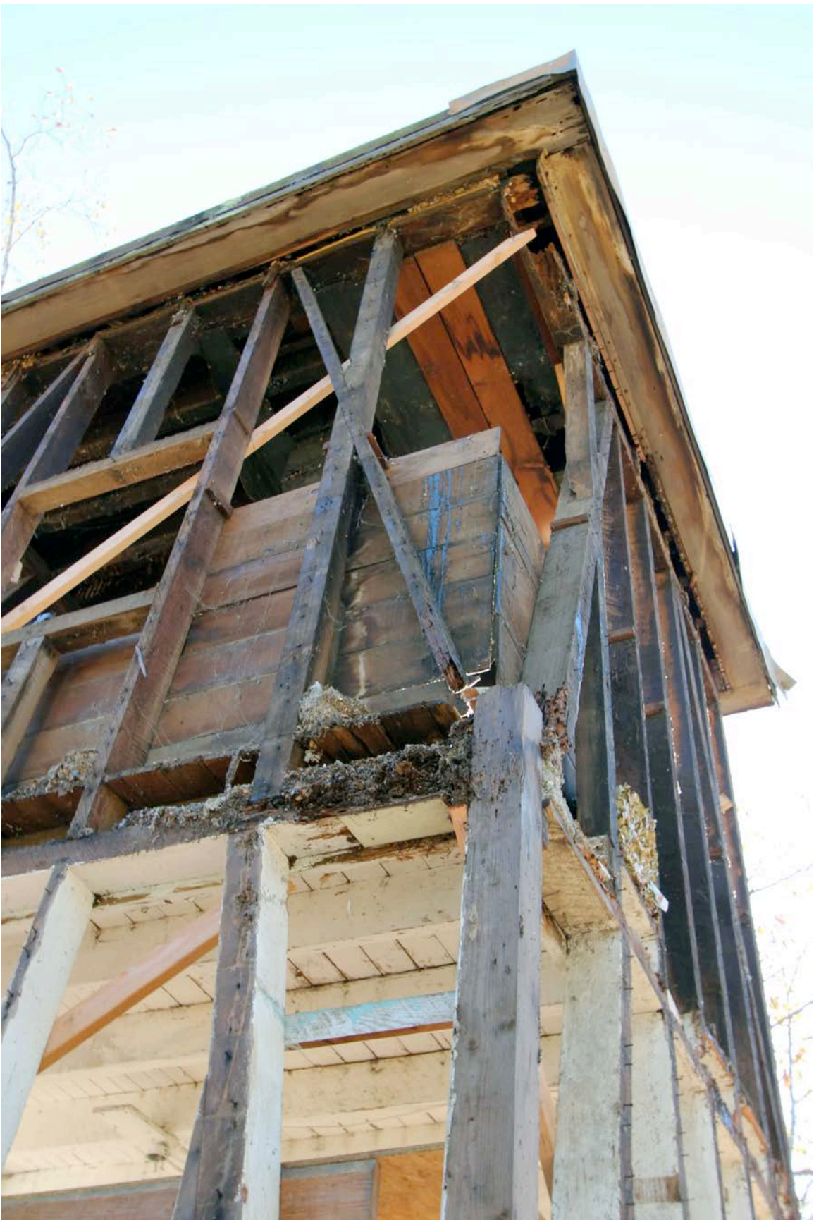
Plate 19. Deteriorated tower structural members.
