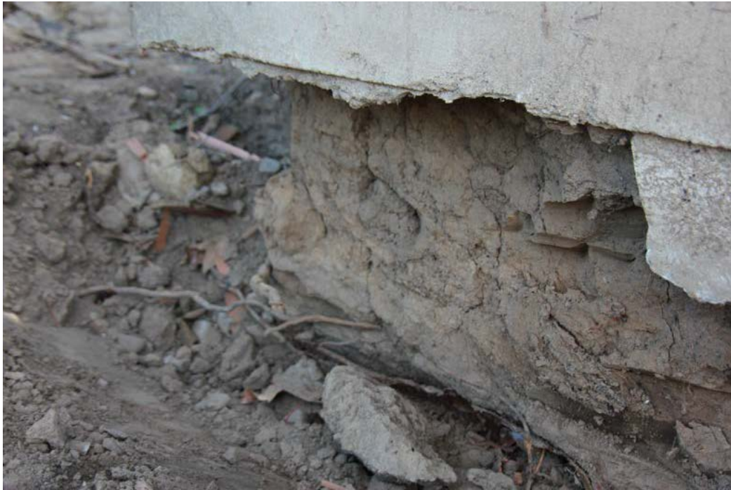
Plate 8. Deteriorated adobe walls at foundation. November 2013.
