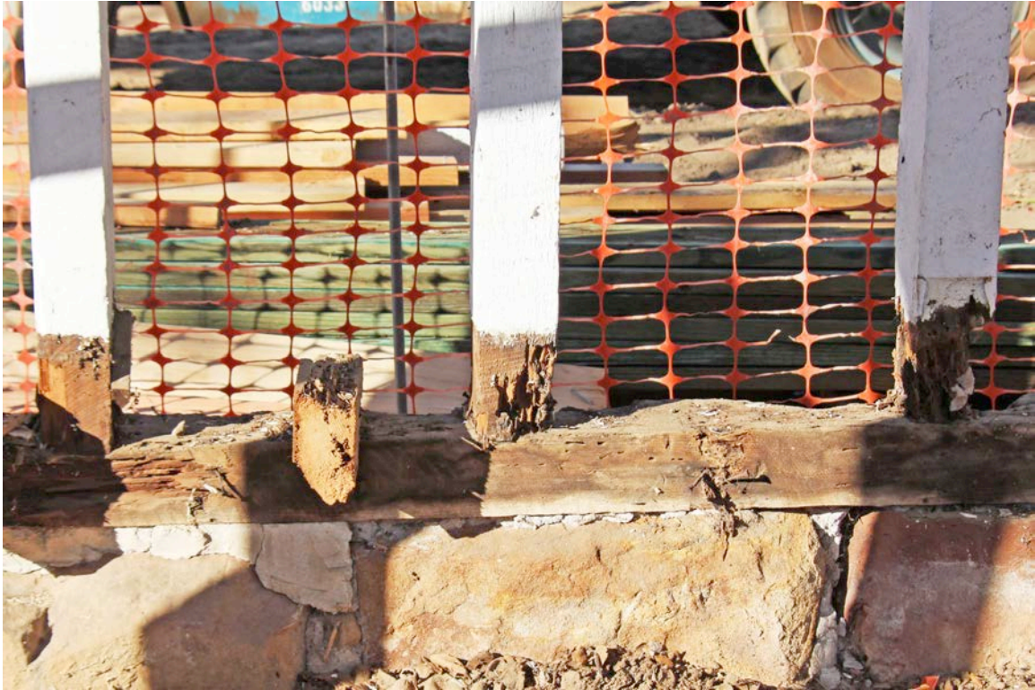
Plate 20. Deteriorated tower structural members resting on stone foundation.
