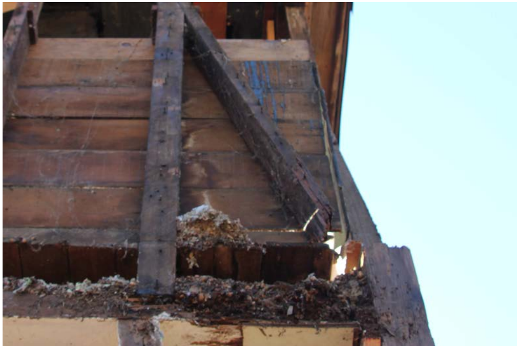
Photo 6 : Rot at upper floor where cross bracing meets floor plate. Corner post completely gone.
