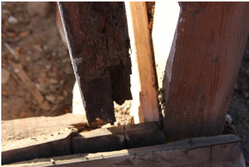
Photo 8 : Connection of brace post to sill plate completely rotted away
