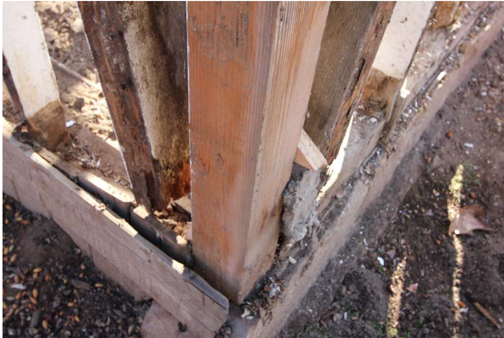
Photo 9: Stone Foundation at Tower on right, earth to wood contact on left
