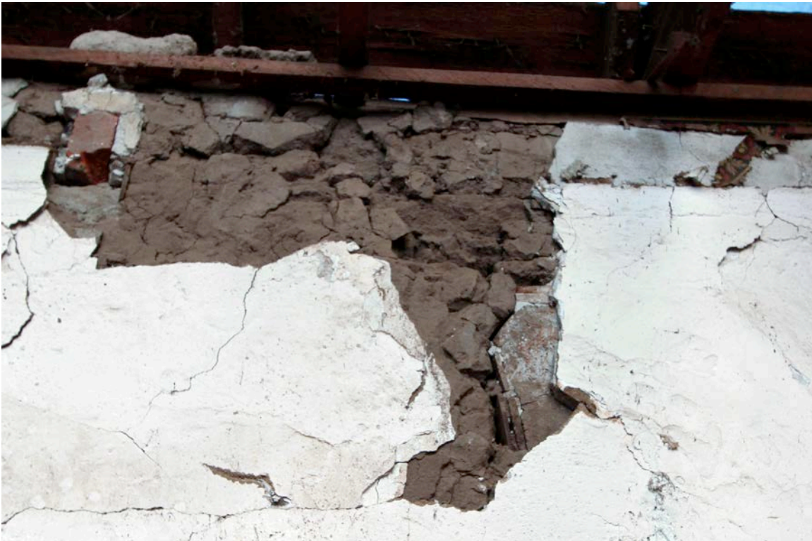
Plate 10. Upper adobe wall showing crumbling blocks. November 2013.
