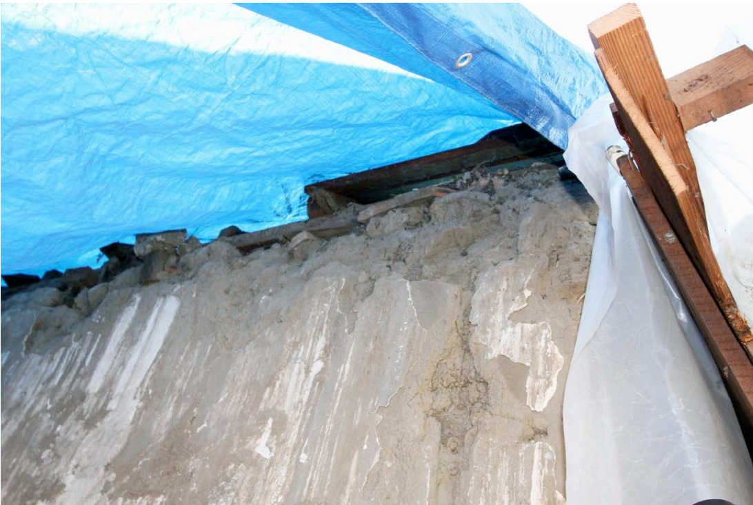
Plate 12. Crumbling blocks at the roof line. November 2013.
