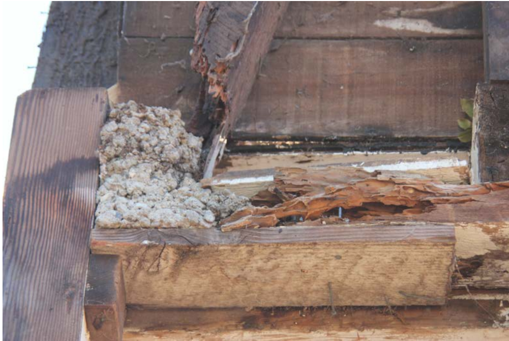
Photo 7 : Rot at key structural connection
