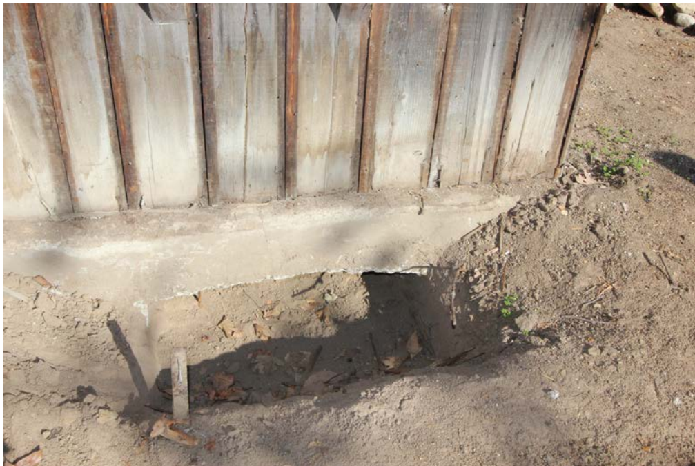
Photo 10: Excavation at perimeter of slab at Cottage showing the absence of a footing
