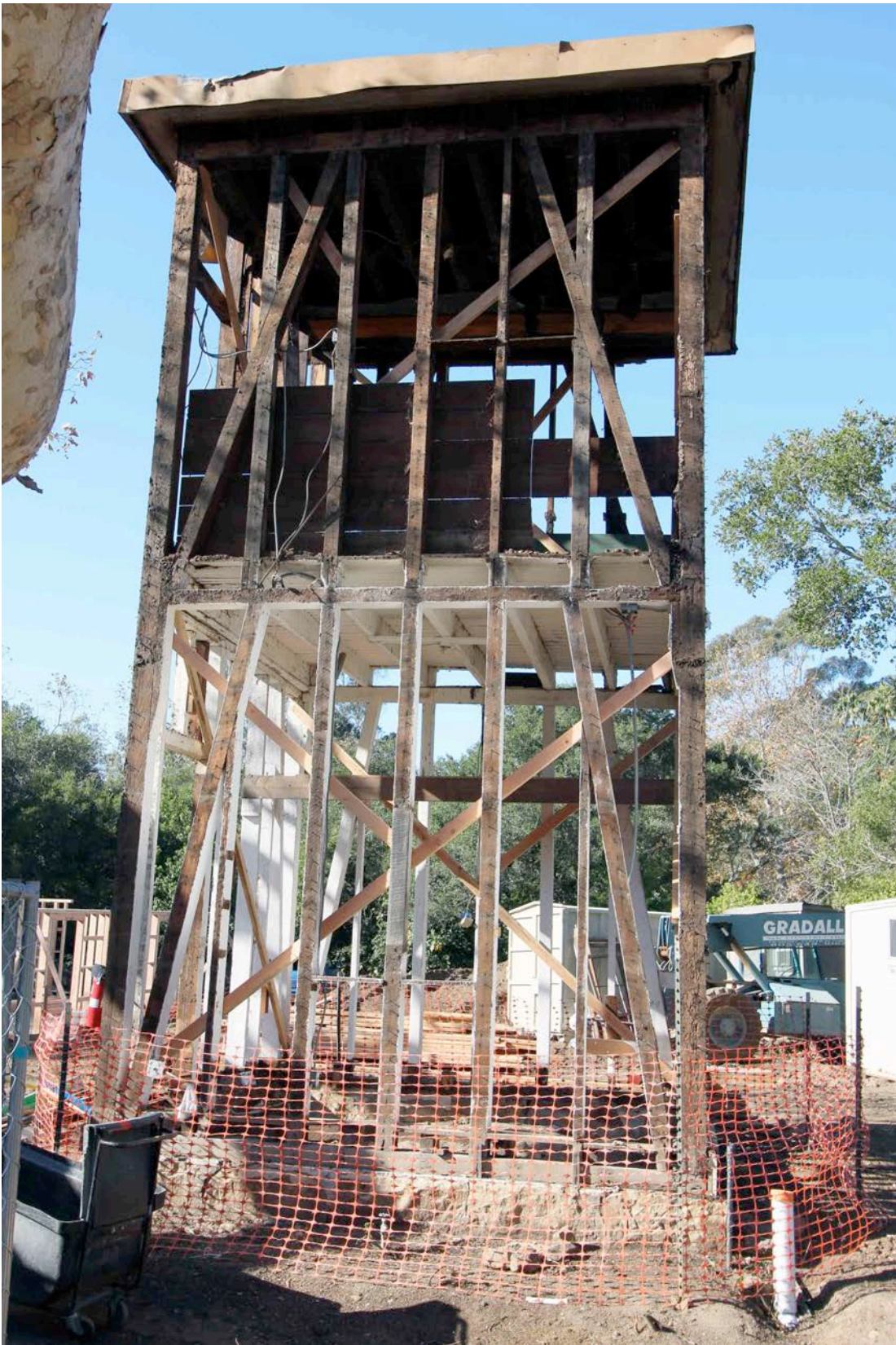
Plate 18. Tower showing deteriorated structural members.
