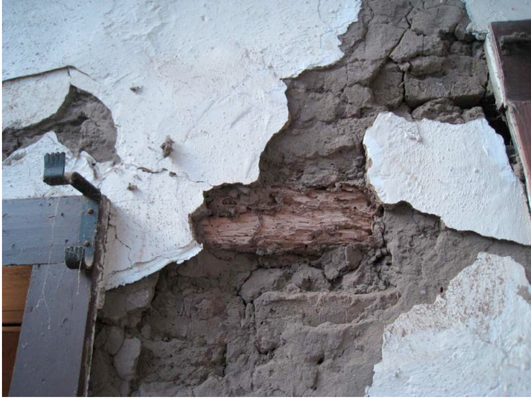
Plate 9. Detail of adobe west wall showing dry rot in structural wood member. November 2013.
