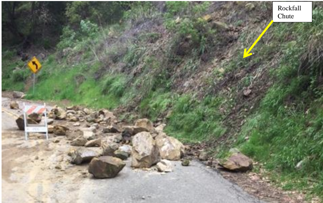
View of East Mountain Drive, looking north, showing rockfall from intense prolonged rain events in February 2017. The embankment slope above the roadway was denuded of vegetation as a result of the Thomas Fire and experienced rockfall events as a result of the fire and the debris flow that followed.
