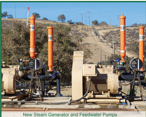
New Steam Generator and Feedwater Pumps
