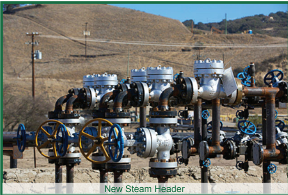
New Steam Header
