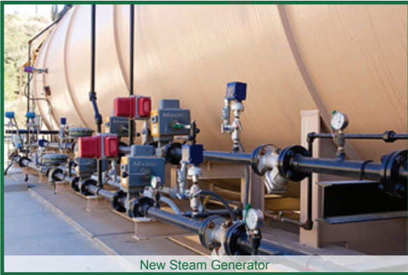
New Steam Generator
