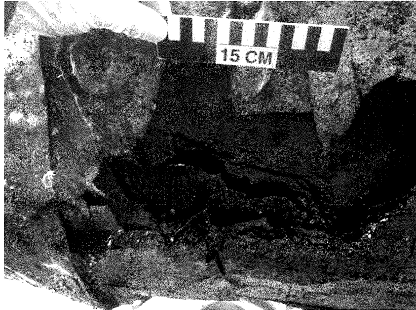
Figure 4. The failed pipe and surrounding insulation and coating.
