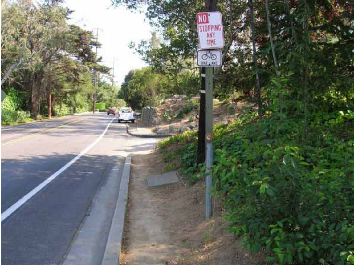
Figure 3: Roadside environment with multiple encroachments.
