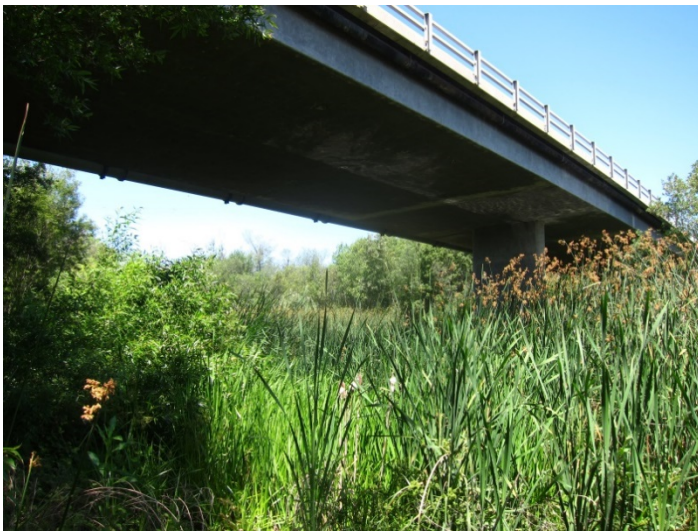
Existing Floradale Avenue Bridge No. 51C-006 over Santa Ynez River looking downstream and to the northwest
