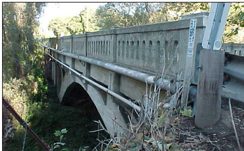
View of Rincon Hill Road Bridge No. 51C-0039, looking north along downstream edge of bridge
