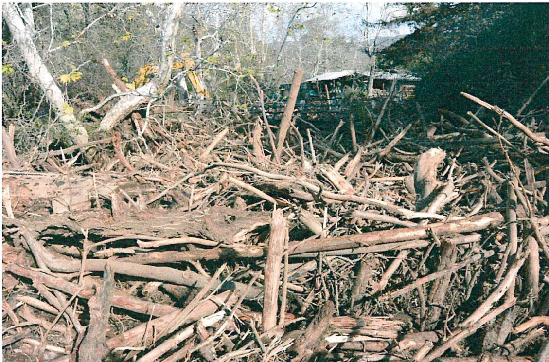
Figure 8: Coarse woody debris clogging the lower El Capitan Creek Bridge
