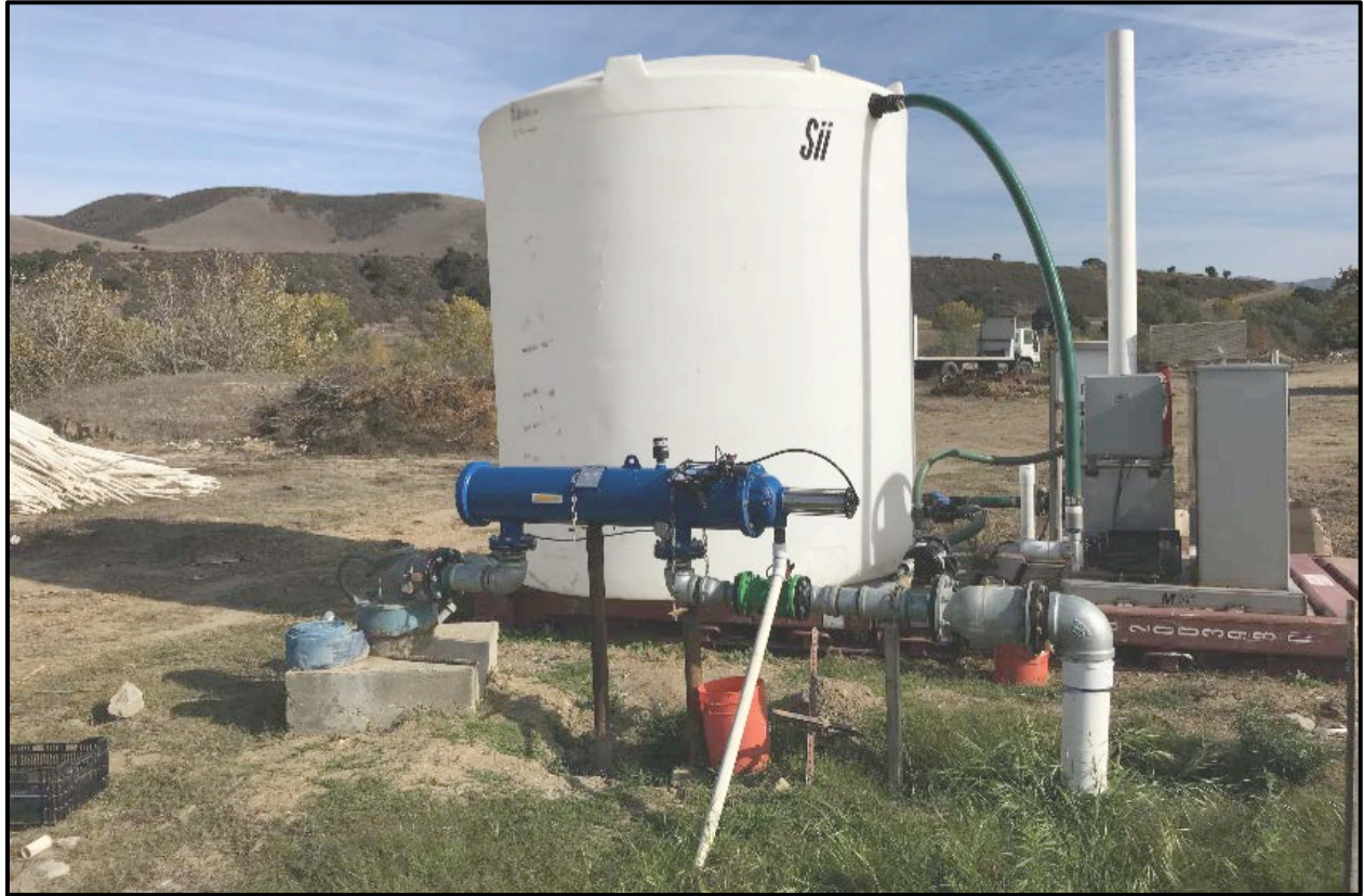
Photo 1. The shallow alluvial water well at 5645 Santa Rosa Road.
