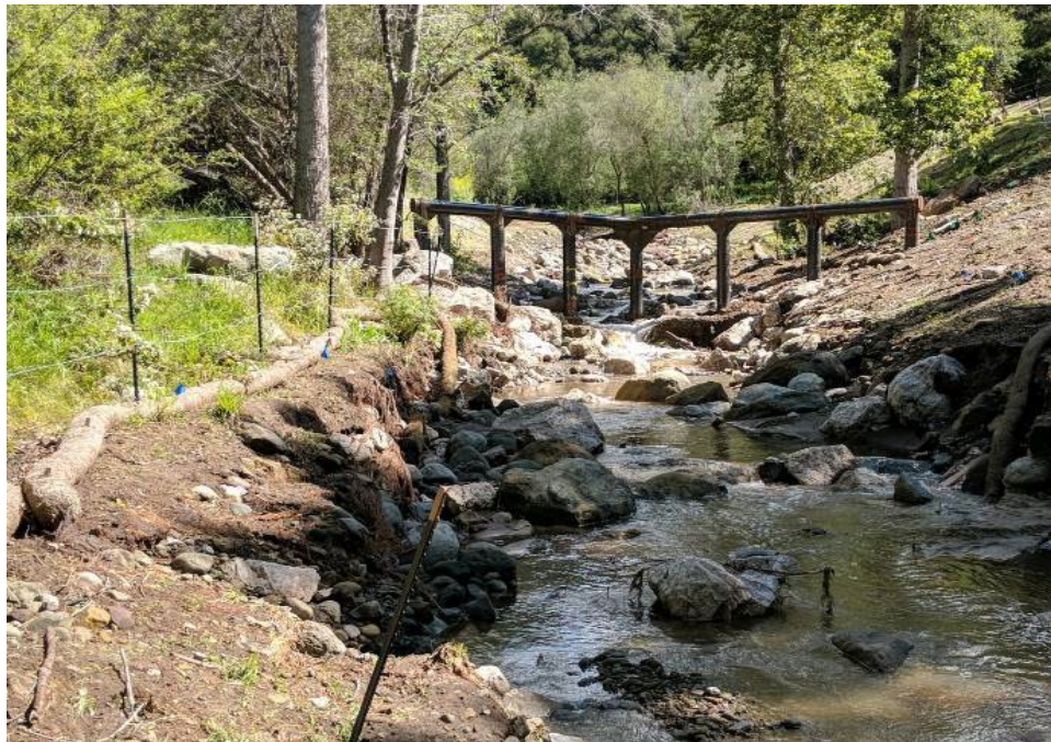
Photograph 4.5-3: Maria Ygnacio Creek Temporary Debris Rack
