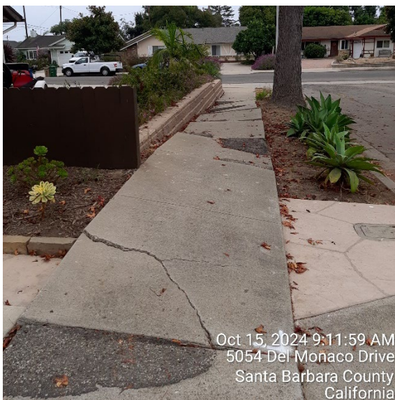
Figure 1: Typical Location of Hardscape repairs – San Domingo Dr
