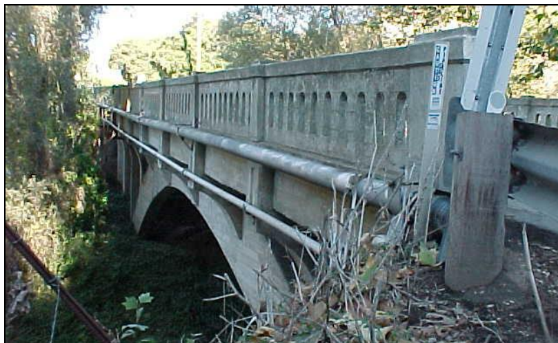
Rincon Hill Road Bridge No. 51C-0039 from the southwest corner of the structure
