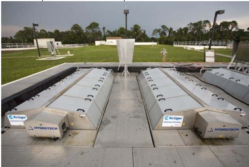
FIGURE 3-7 A Full-Scale Hydrotech Disc Filtration Facility
