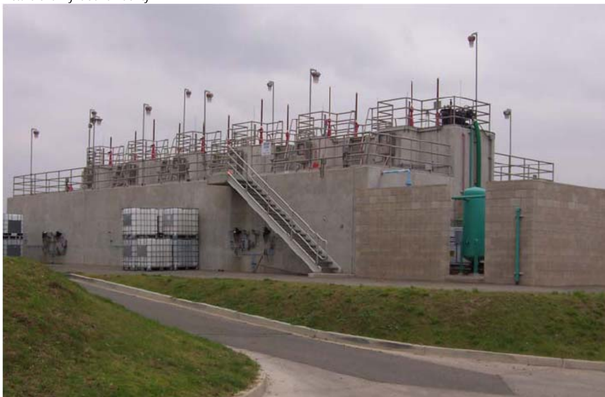
FIGURE 3-6 Picture of a DynaSand Facility
