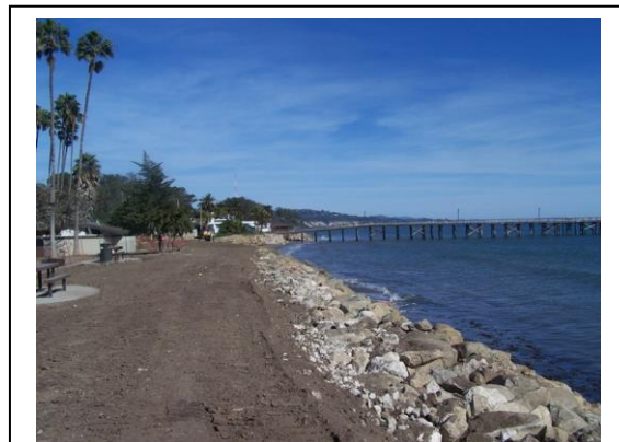
In halting landward erosion of Goleta Beach Park, under current severe beach erosion and historically low sand conditions, new and existing revetments have contributed to Goleta Beach becoming intertidal. The duration of this condition will depend substantially on renewed sediment input into the system
