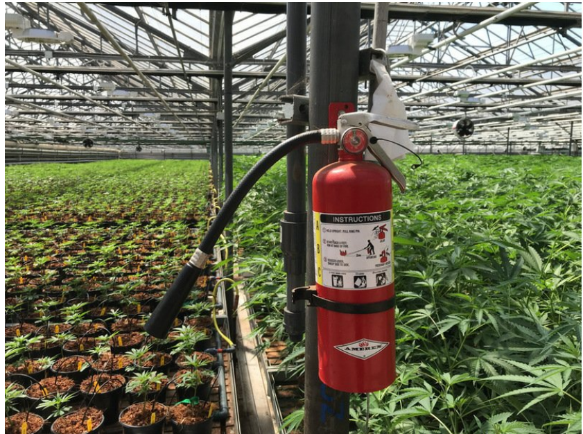
Fire extinguisher has been discharged and the tag is missing.
