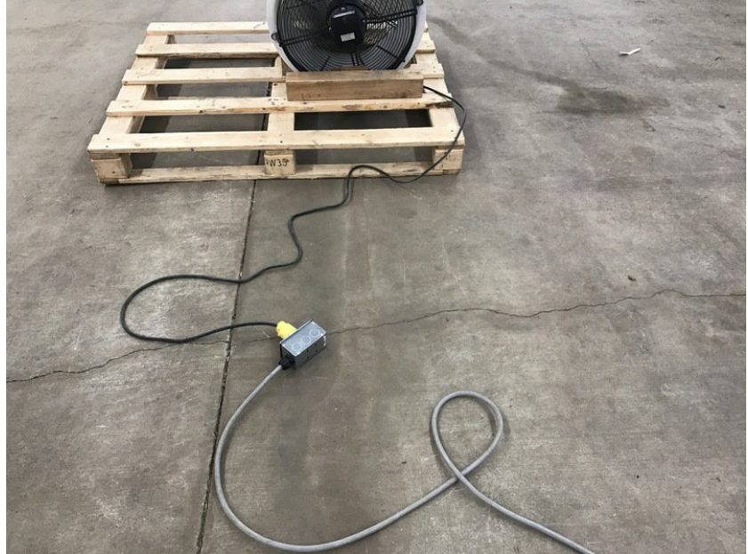
"Home made" extension cords not permitted.
