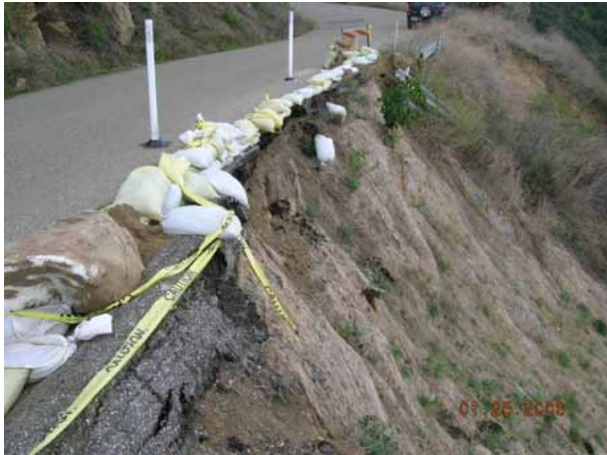
Photo: Post-storm Conditions at M.P. 2.28 (Site 1T38)
