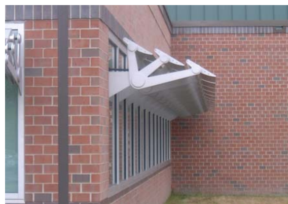
Figures 2-12 and 2-13. U.S. EPA New England Regional Laboratory, Chelmsford, Massachusetts (LEED Gold Rating, Version 1.0) Reflective light tubes, with diffusers designed to fit suspended ceiling systems, and exterior light shelves bring daylight deep into the building. (Photo: Don Horn)
