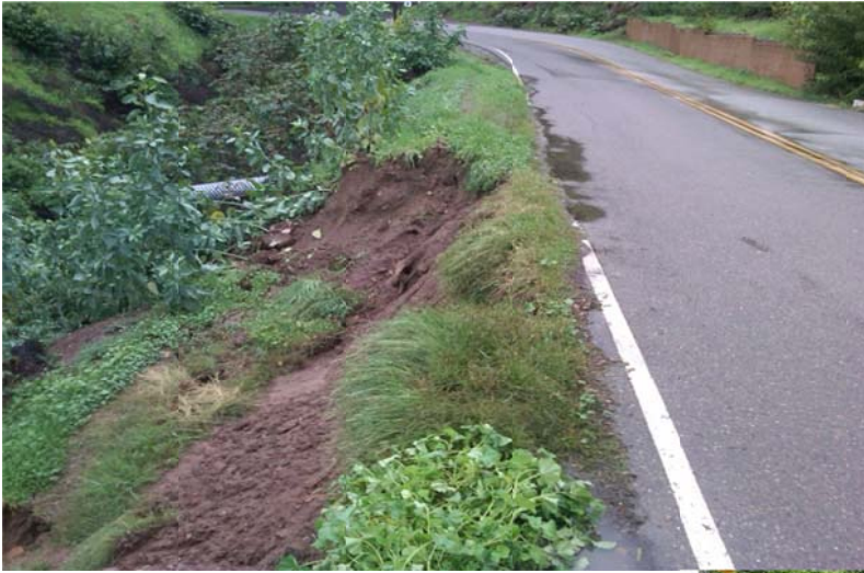
Reduced shoulder width at Tunnel Road MP 0.7 (Site 1A02)
