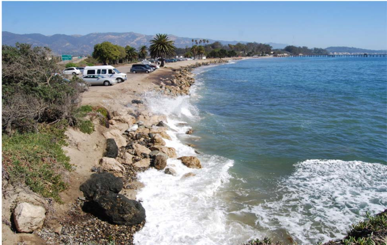
Exposed revetment at Goleta Beach on October 18, 2016, courtesy Surfrider Foundation.
